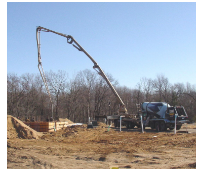
30 ft. cement pump (used when access difficult for cement truck) pours foundation for one of the duplexes being built.
